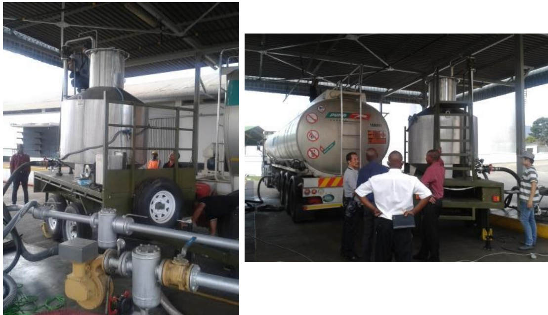
Picture 1; Commissioning of prover tank system
